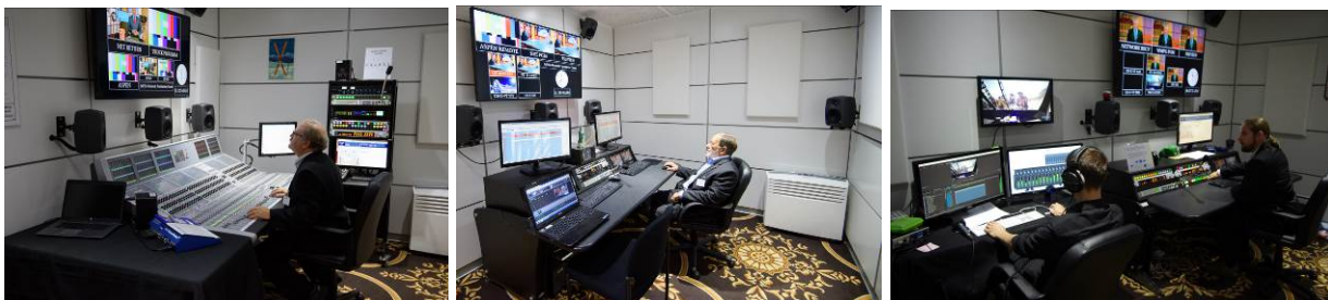
Figure 1. Professional rooms of the test bed: Remote Truck, Network Operations Center, Local Affiliate (l to r)
